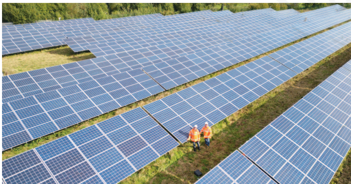
1.9 MW, Testwood Water Supply Works solar farm, Peel Common, Hampshire, UK.
