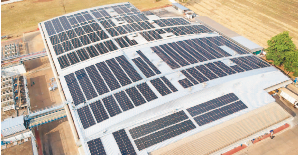
Solar PV installation on the site of agro-industrial company Cargill in Thailand.
