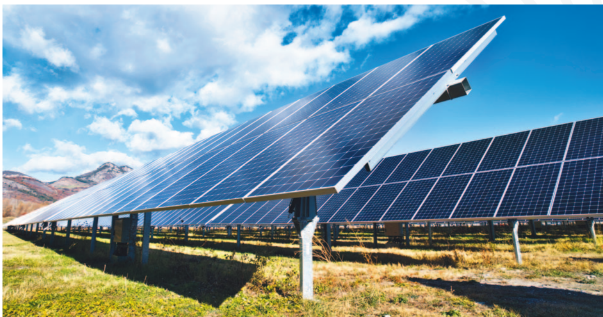
15 MW, Curbans, France.
