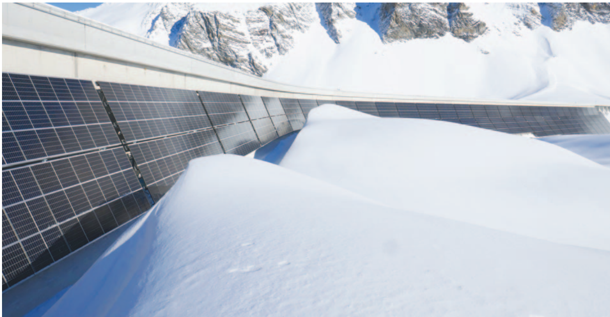
2.2 MW alpine solar plant at Muttsee, Switzerland.
