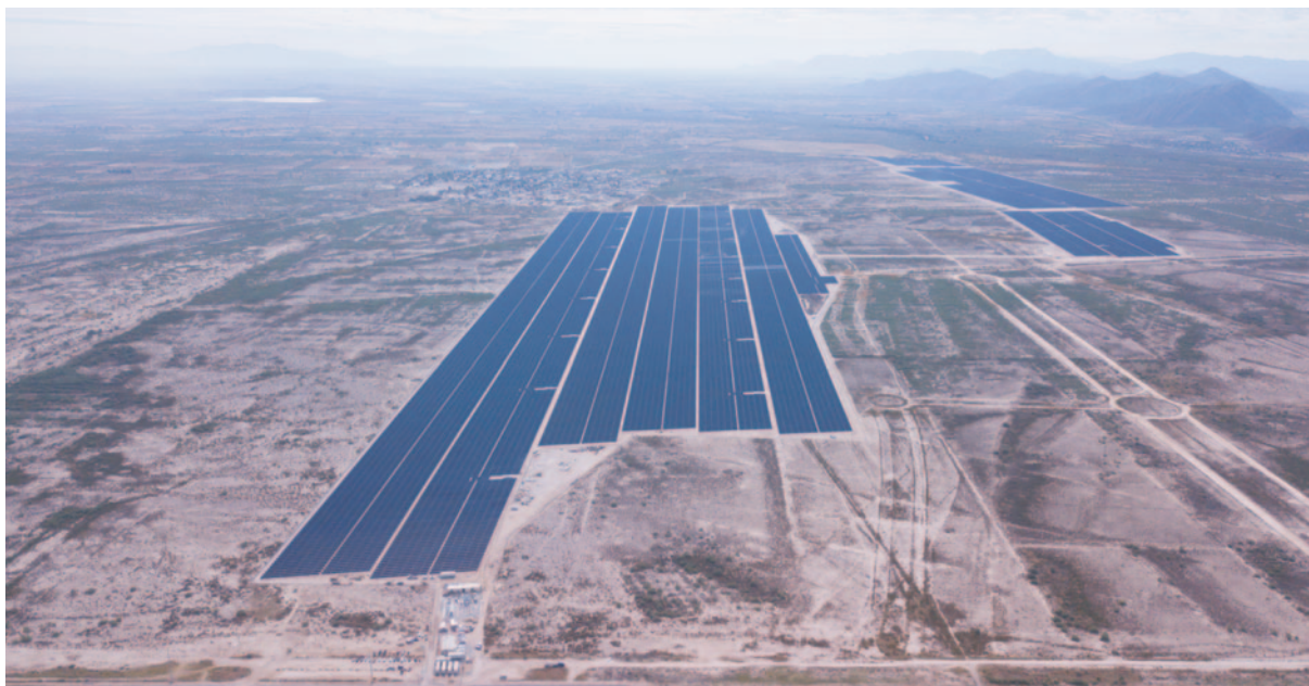
101 MW, Laguna solar park, Matamoros, Coahuila, Mexico.
