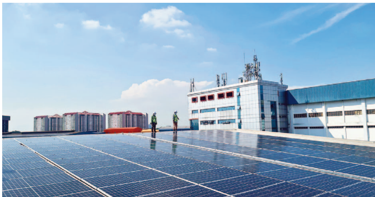
312 kW on-site solar PV system in Shah Alam, Malaysia.
