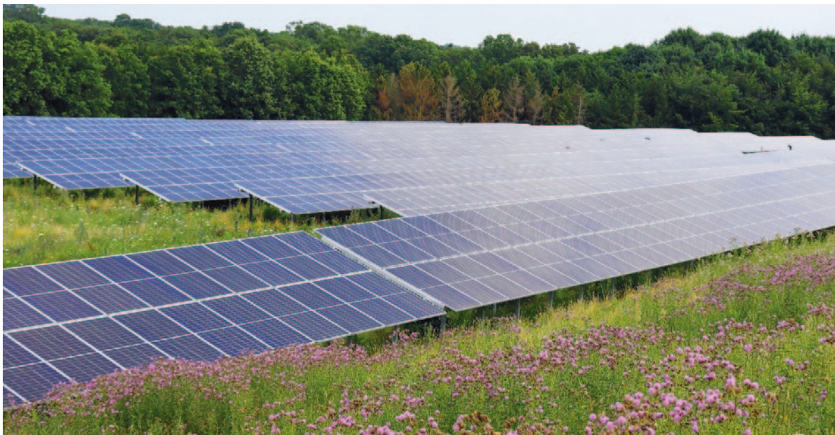
8.9 MW, Armhoede solar park, built on a former landfill.
